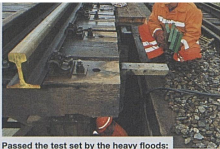
Passed the test set by the heavy floods: lift-up of a bridge in the Valais
