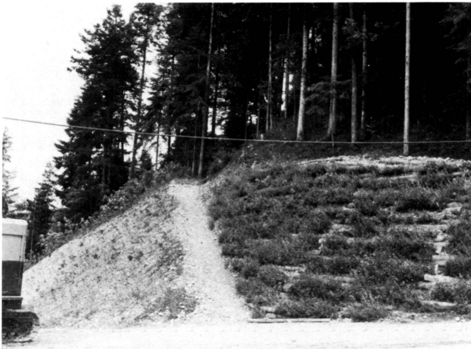
Signau, Hangrost angewachsen. Signau, grille au début. Signau slope grid in the process of becoming overgrown.
