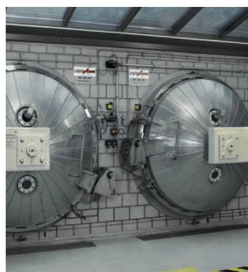
Papersave swiss plant, Wimmis. Both chambers are closed. The plant is in operation.
