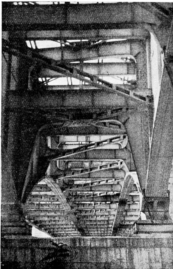
Fig. 2. View of the steel construction of the Arpád-bridge showing welded elements from underneath.
