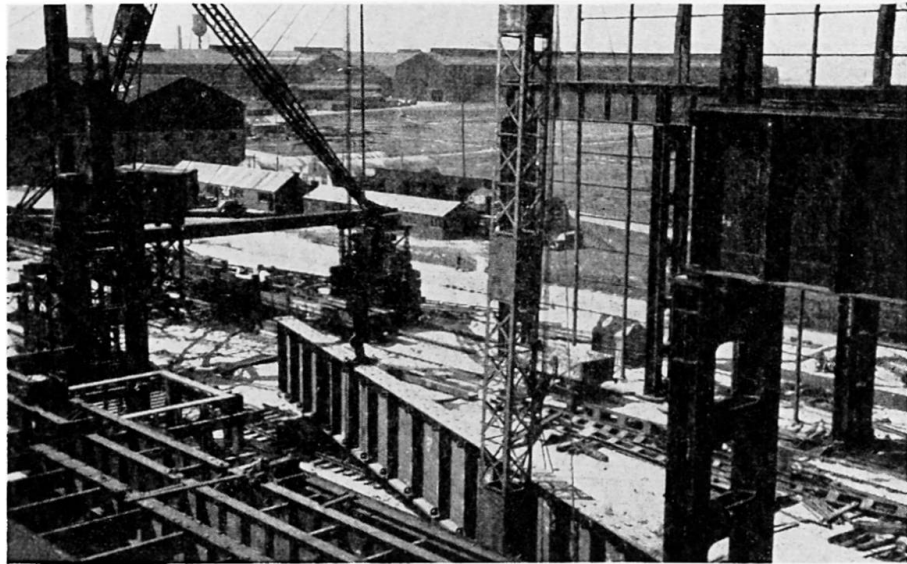
Fig. 10. 100-ton welded girder being lifted by a derrick crane and a derrick mast
