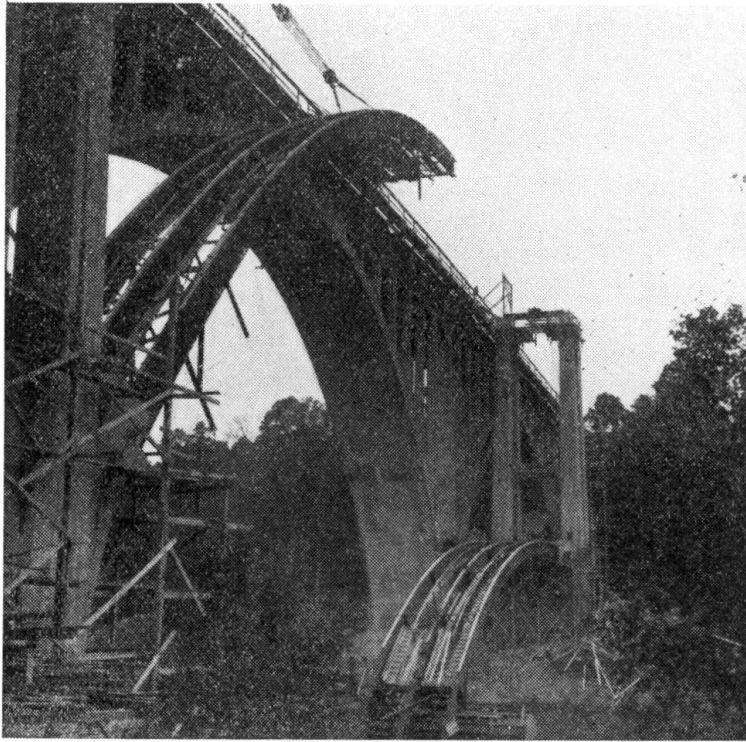
FIG. 6. First part of the arch in its final position, the second being hinged at the abutment
