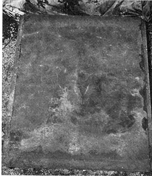
Fig. 10. The 9 ft. By 7 ft. Deck Plate After Removal of the 1\frac{1}{2} -in. Surfacing. Note Absence of Any Corrosion After 4\frac{1}{2} yr., Due to Cracking; and Also the Very Considerable Corrosion Where the Mastic Asphalt Had Not Adhered Properly Over the Front and Centre Portions of the Plate.
