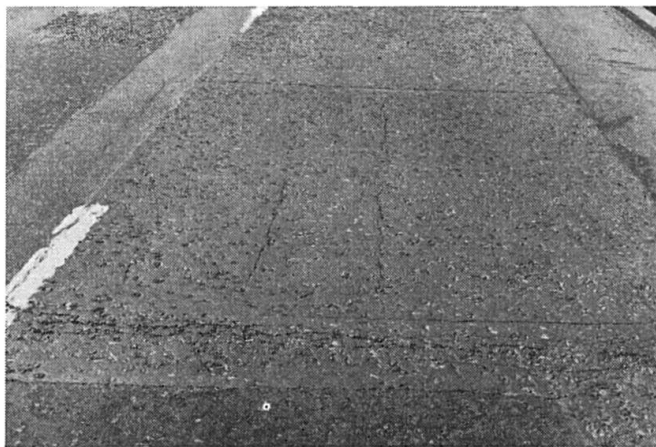
Fig. 8. General View of Bridge Panels After 2 1 / 2 yr. with 1-in. Surfacing in Foreground. Note the Pronounced Cracks Over the Three Central Stiffeners and Incipient Cracks Over the Outer Stiffeners.
