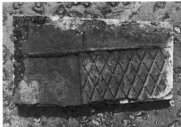
Fig. 3. The Underside of the 1½-in. Surfacing Removed From the Junction of the Smooth and Chequered Plate Panels.
