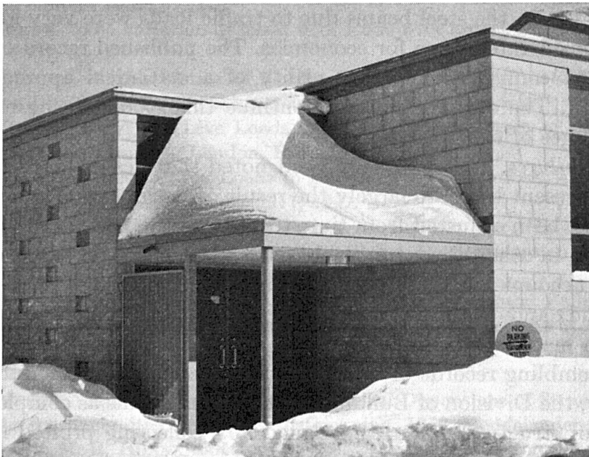
Fig. 3. A Triangular Snow Accumulation (Maximum Load 80 lb./sq. ft.) Resulting From Wind Action on a Building in an Area with a 50 lb./sq. ft. Design Load.
