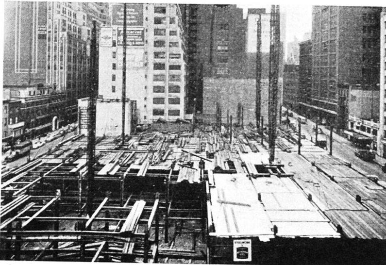
Fig. 13. With several derricks erecting, staggering the time of jumping results in better delivery of steel. Working floors should be completely planked for safety.
