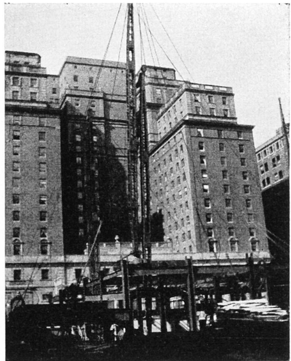
Fig. 7. To jump guy derrick, boom is separated from mast, guyed as a pole to lift mast to upper floor. Mast then picks boom up to itself.
