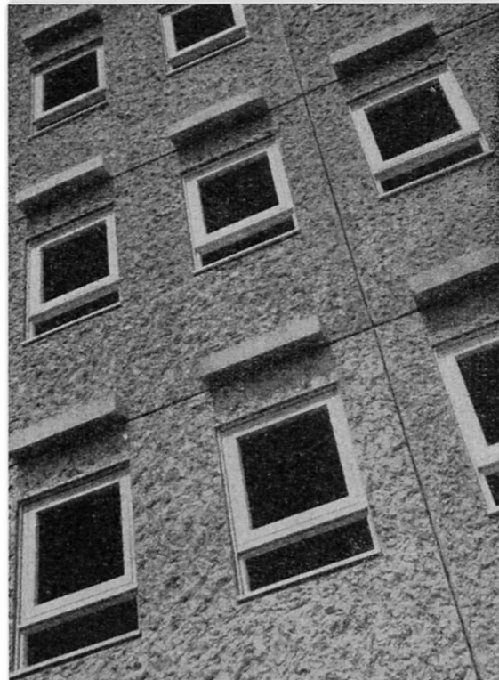
Fig. 1 - 20-storey block of flats at Smethwick of precast load-bearing walls with simulated rock finish.
