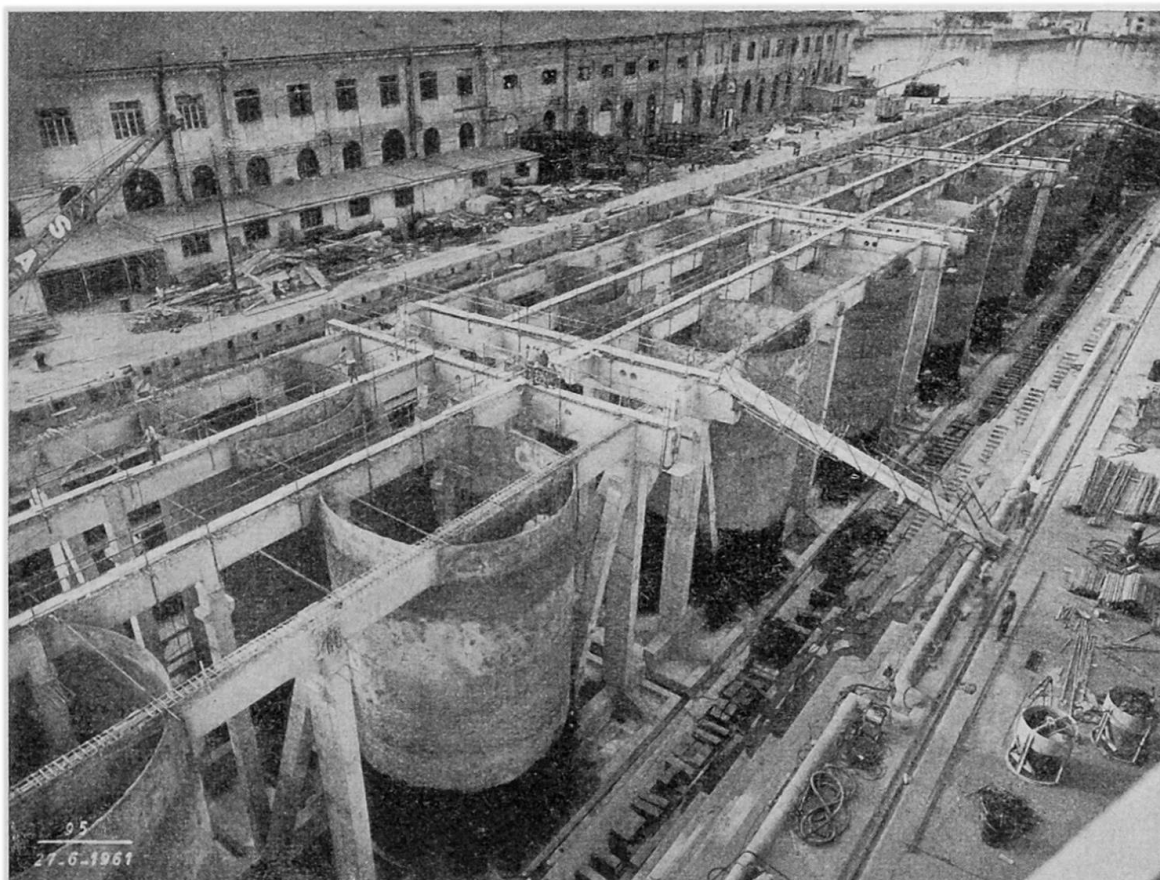
Fig. 13 - Edisonvolta thermal power plant, La Spezia. In-situ prefabrication of the fuel discharging wharf (Impresa SALCI).
