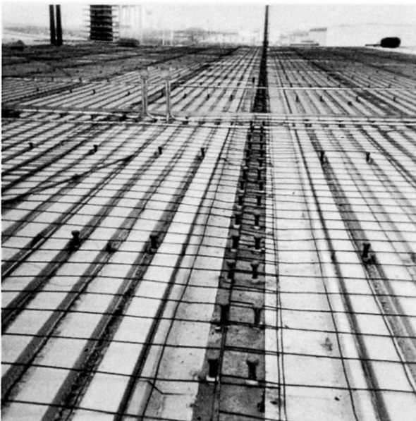
Fig. 13. Category II(b) Form – Overview showing composite beam and girder construction. (Note temperature steel.)
