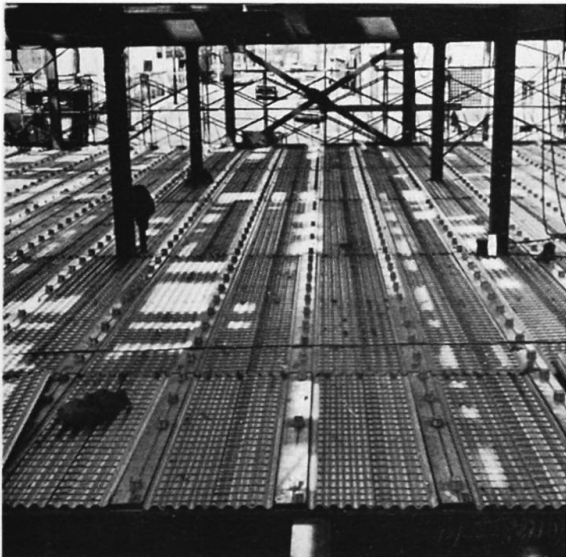
Fig. 9. Category I Form — Overview showing all forms and raceways with service fittings in place.
