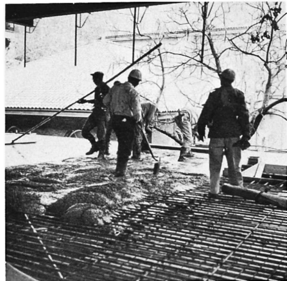
Fig. 10. Category I Form — View showing placement of concrete. (Note negative reinforcing bars.)
