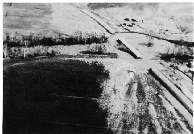
Figure 3 End scour after waterway blockage.
