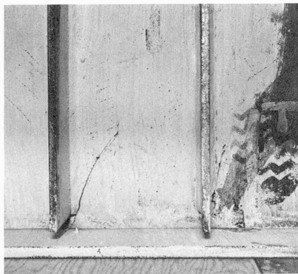
Fig. 7. Typical Failure at Web Stiffeners.
