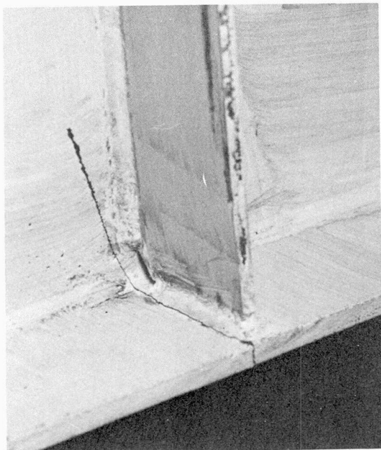
Fig. 2. Typical Failure at Stiffeners Welded to Web and Flange.
