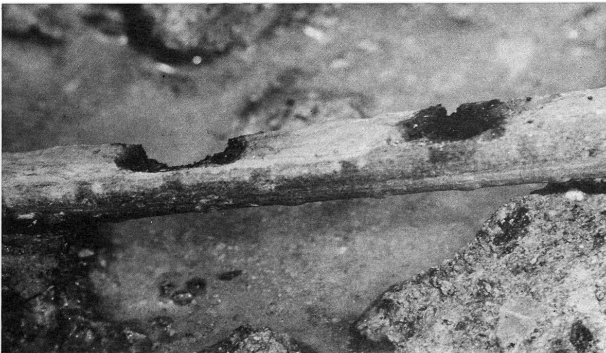
Localised corrosion on steel in concrete
