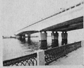
Bridge over the River Moscow Concrete continuous girder with spans 62 + 114 + 62 m (for combined traffic of city vehicles and Metro trains)
