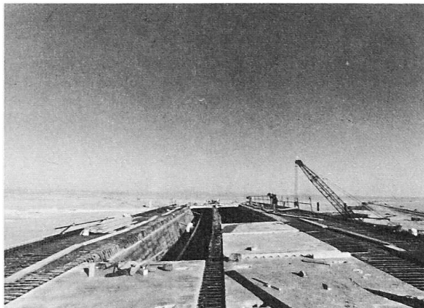
Fig. 4 Placing of the precast deck slab elements after concreting bottom slab and webs and applying a partial prestress
