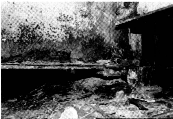
Fig. 1 An example of corrosion
