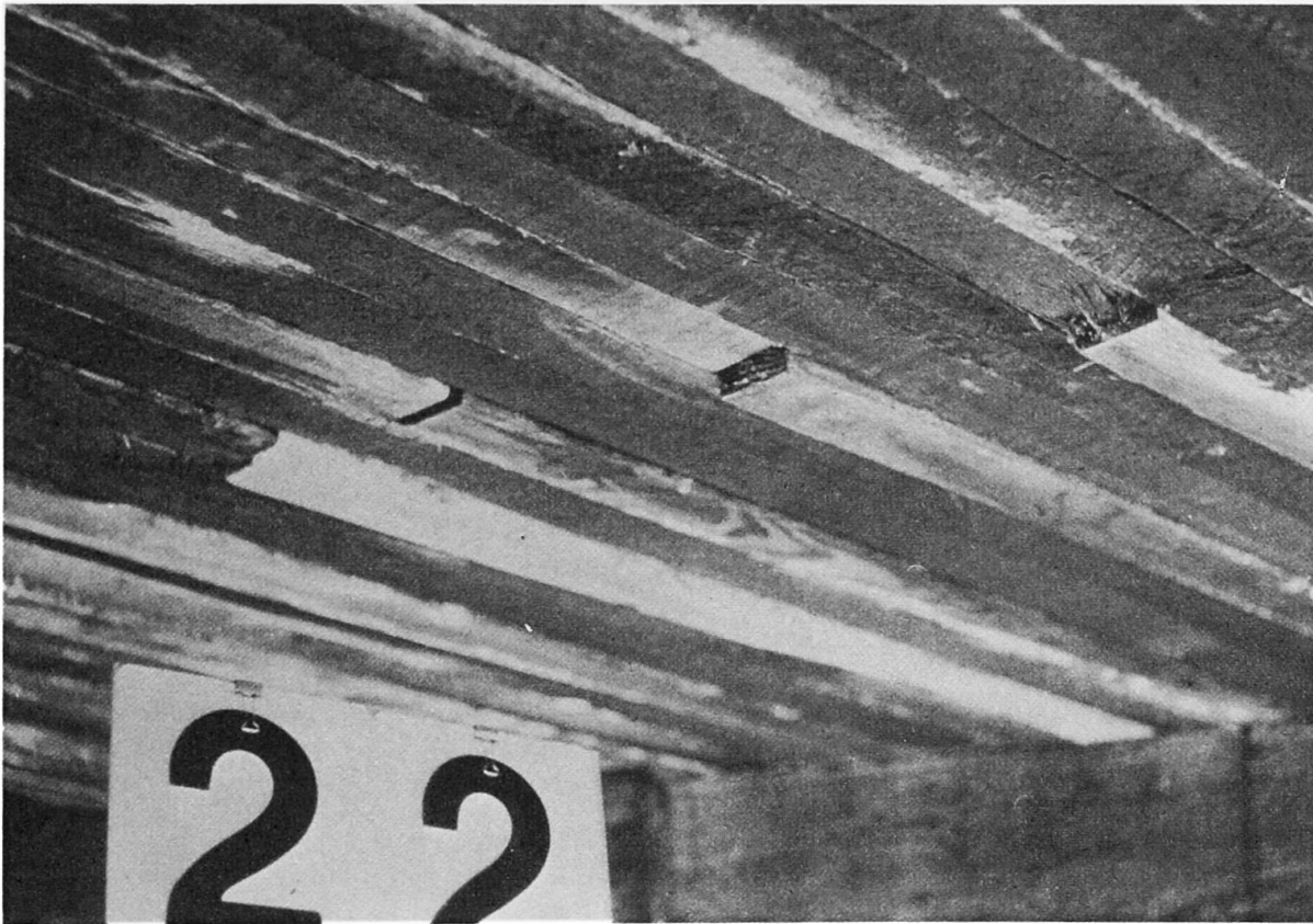
Figure 12 "Piano-Key" Failure of Nailed Decks with Butt-Joints
