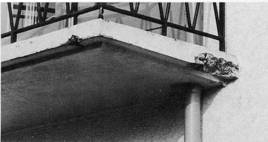
Fig. 6 Corrosion damage due to carbonation
