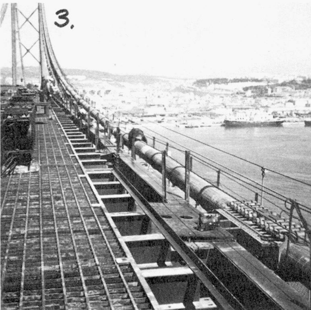
Photograph 3 shows some additional details of the grid floor which will be filled with concrete.
