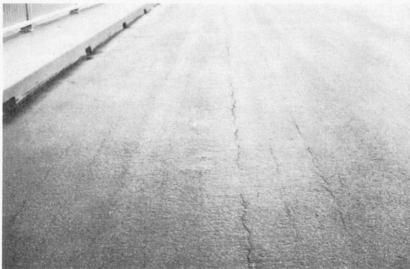
FIGURE 4. LONGITUDINAL CRACKS IN THE ACPAVEMENT ON THE CONCORDIA BRIDGE AFTER TWO YEARS IN SERVICE
