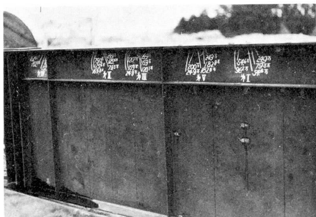
Fig. 11. Location of Cracks Type BM-1 in Girder F-5.
