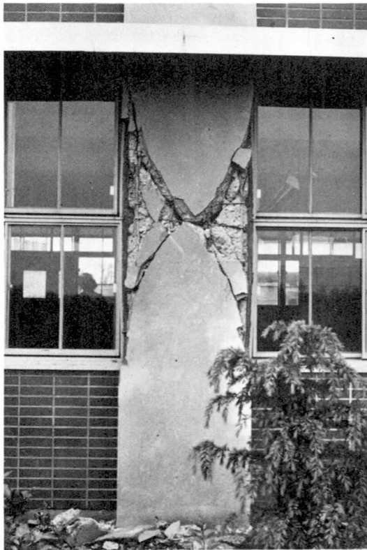
Fig. 2 Shear Failure in a Column
