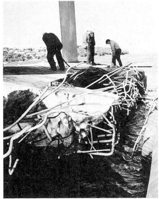
Fig. 5 Damage to Pile Cap 20
