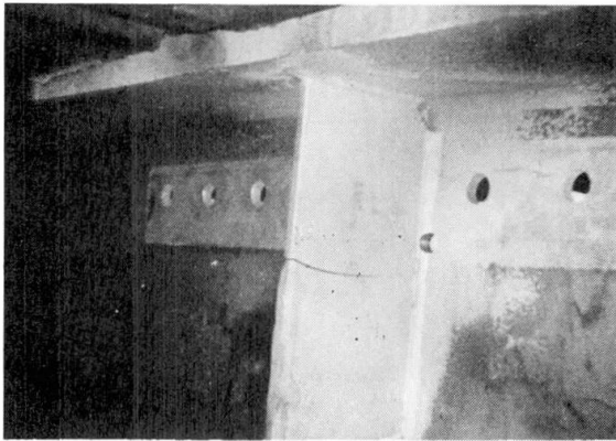
Fig. 11 Hole at Stiffener
