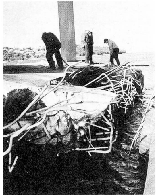
Fig. 5 Damage to Pile Cap 20
