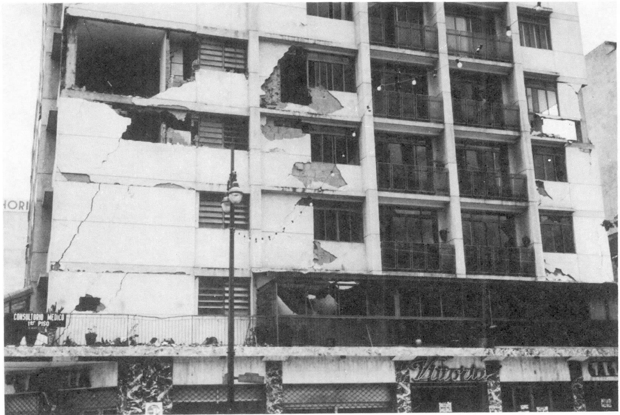
Fig. 10: Damage to nonstructural elements in 1967 Caracas, Venezuela earthquake
