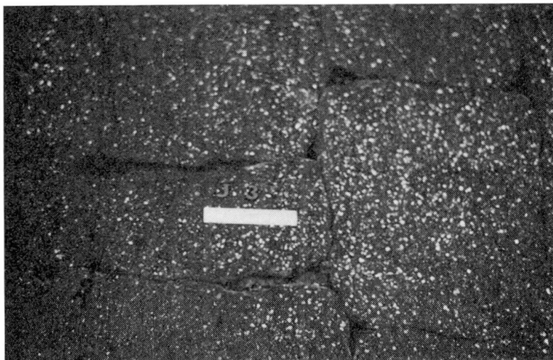
Fig. 3 Severe Cracking of the Surfacing
