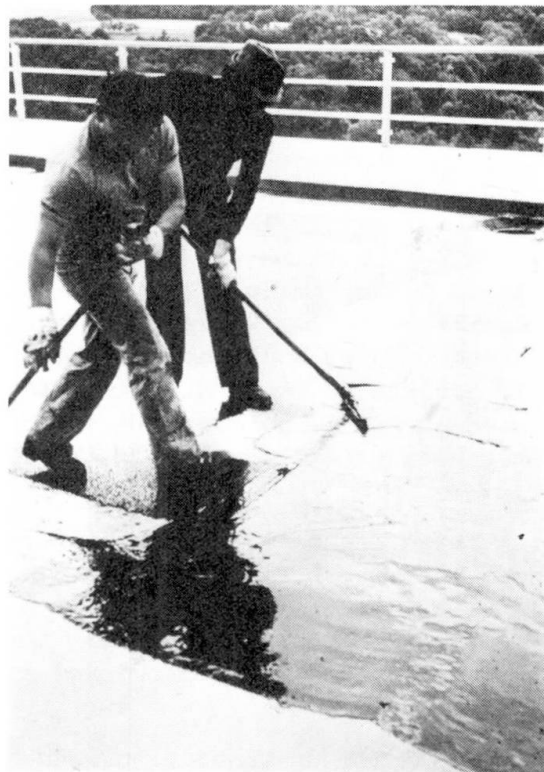
Fig. 21 Spreading of the bitumen epoxy resin waterproofing by hand (bridge over the Kocher valley at Geislingen)
