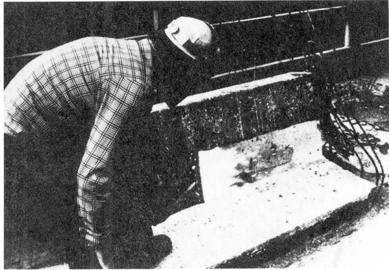
Fig. 22 Flame-cleaning of carbonated top concrete layer of concrete guard kerbs (valley bridge Pfädchensgraben)
