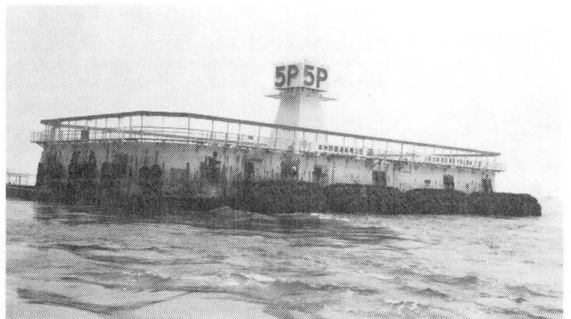
Fig.2 The Protection Installed on the No.5 Pier of the South Bisan-seto Bridge
