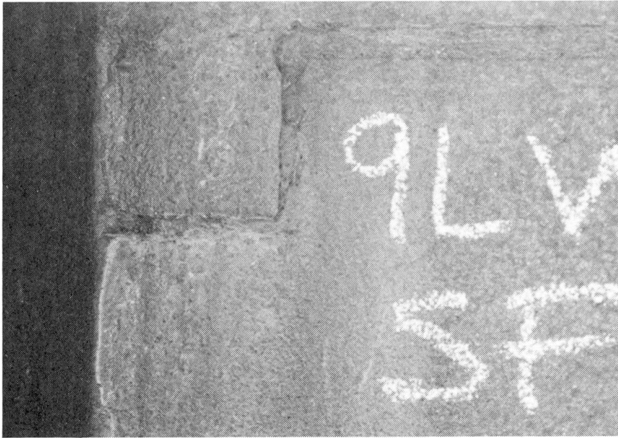
Fig. 9 Cracks at the Cope Closure Plates of a Box Beam
