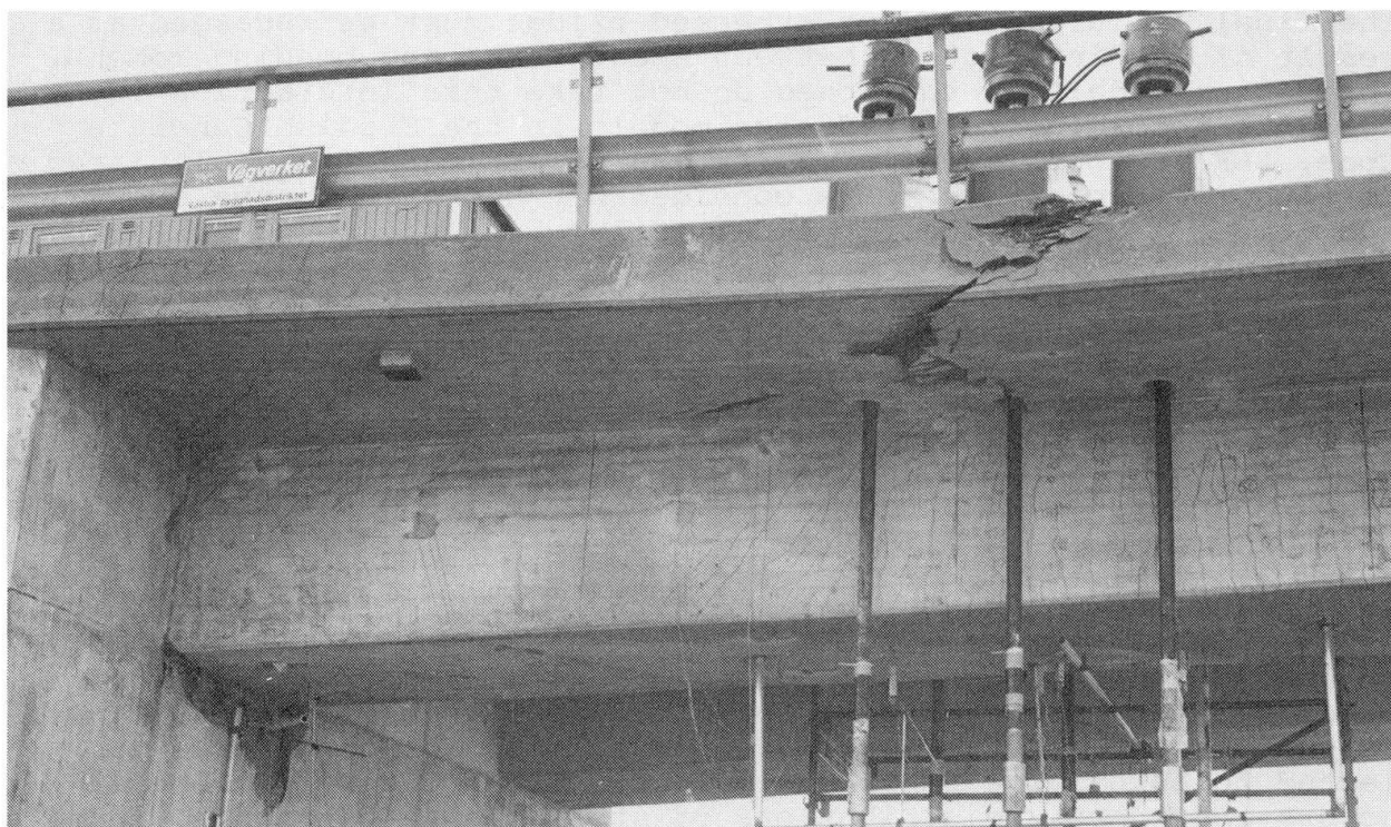
Fig. 7 Failure in the prestressed bridge. Cracking, support failure and concrete compression failure at the top of the loading section can be seen.
