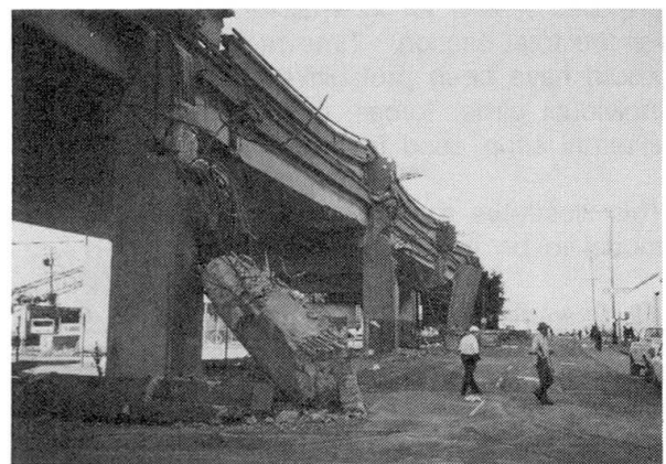
d) PHOTO OF COLLAPSED STRUCTURE
