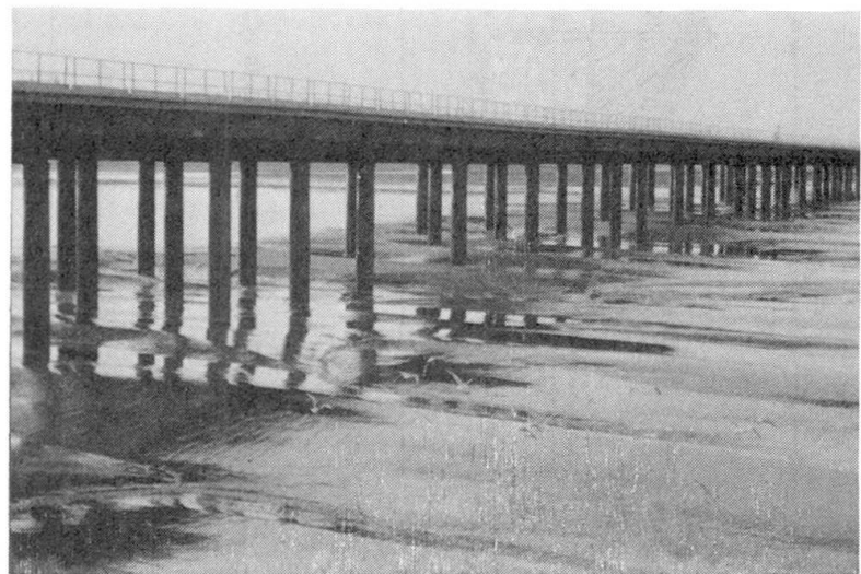
Fig. 6: A photo of the temporary bridge in the swamps at low tide
