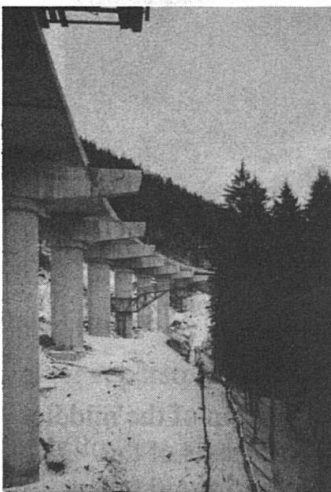
Fig. 4 Destruction outer deck slab
