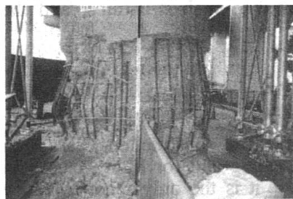
Fig. 2 Bending failure of a RC pier
