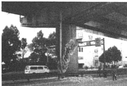
Fig. 1 Shear failure of a RC pier
