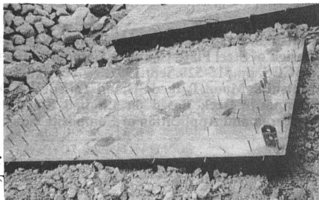
Photo.1 Typical shearing failure of studs
