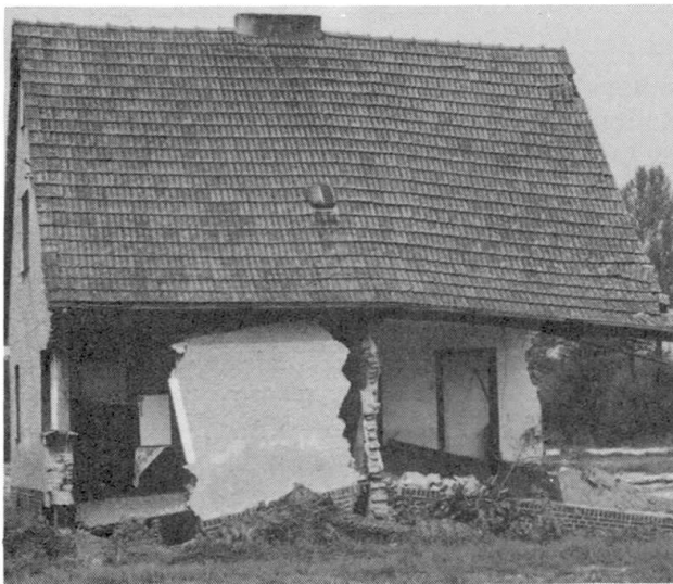
Fig 1. Sudeten development destroyed by the flood in 1997.
