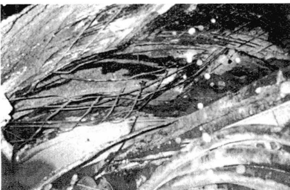
Great Belt Tunnel after a fire during construction.
