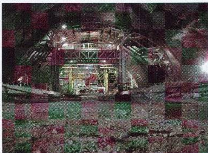
Bétonnage de la caverne de Deriner - Turquie (haut. = 12 m, larg. = 30 m, long. = 120 m)
