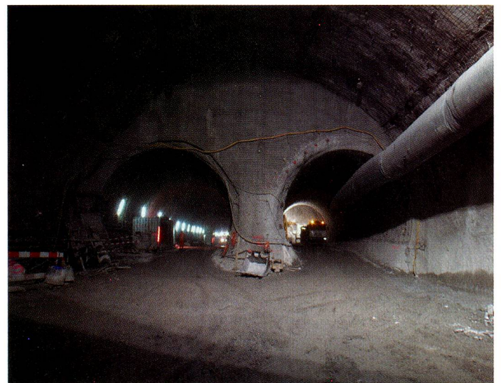
At 57 kilometres, the new base tunnel is the longest railway tunnel in the world.
