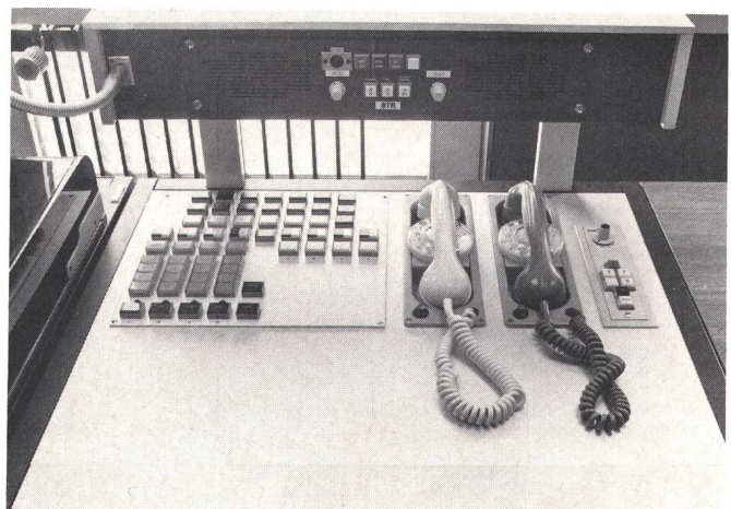
Fig. 6 View of the telephone console
