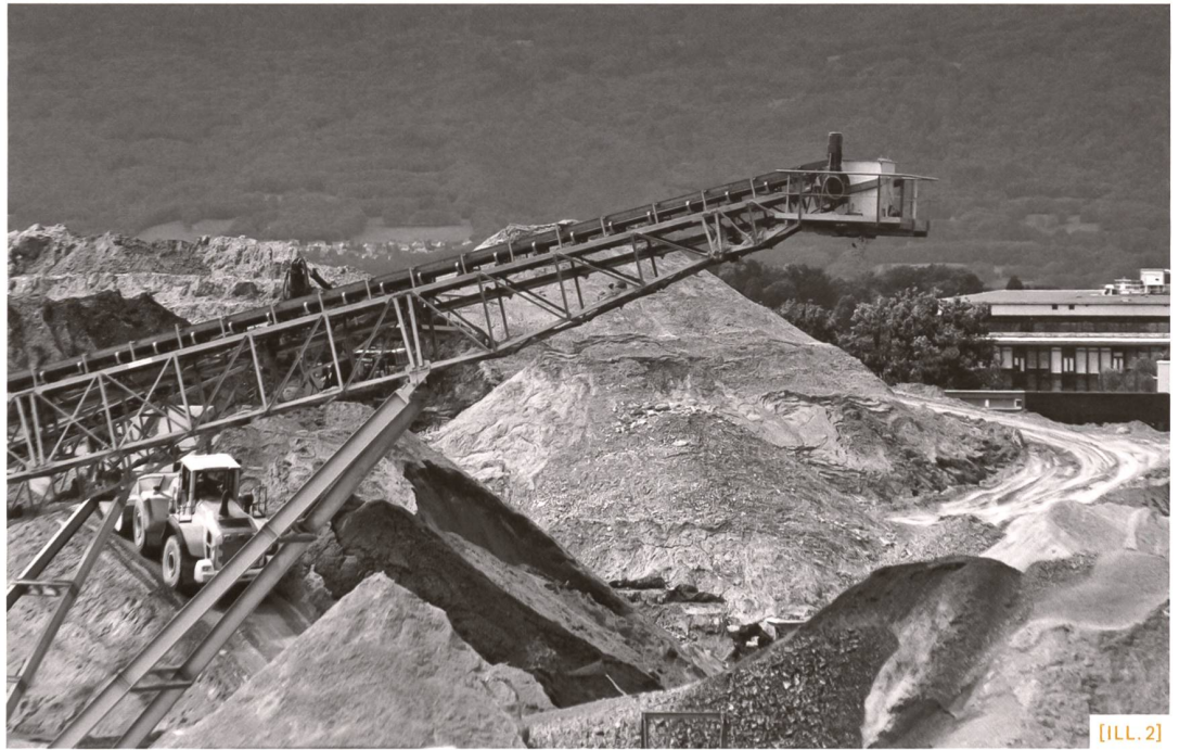
[ILL. 2] ZIMEYSA gravière / Cava di ghiaia ZIMEYSA / ZIMEYSA Kiesgrube (Photo: David Wagnières)
