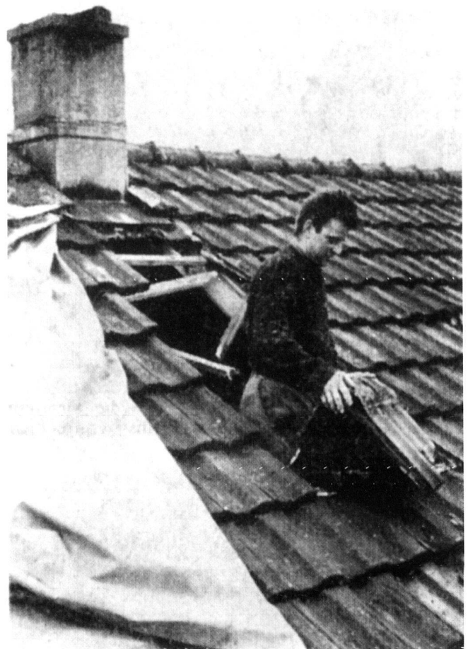
Fig. 7. Sarnen: The top of a chimney destroyed part of the roof (Vaterland, February 18, 1964)
