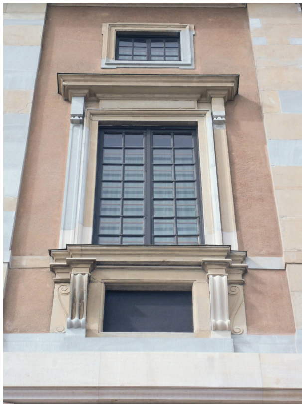
3 The façade after stone replacement. Old Gotland stones are a dark yellowish grey, new Gotland or Roschacher stones are a blueish grey and new Obernkirchener stones are a light yellowish grey. Whether the colour differences are acceptable or not is a matter of ideology and taste (Photo A. Heymowski).
