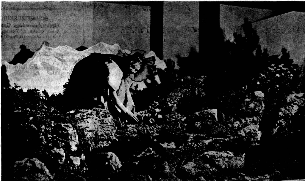
The Alpine Rock Garden at the Swiss Exhibition under Construction. (Photo: Chas. E. Brown.)
